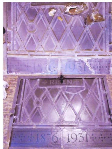
A before and after shot of the window one of the window repairs that took place over the summer. A big thank you to A. Stirling @ Andrew Edward Stirling Stained Glass Repair for his amazing work!
